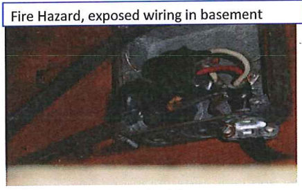
fire hazard. Exposed wiring
